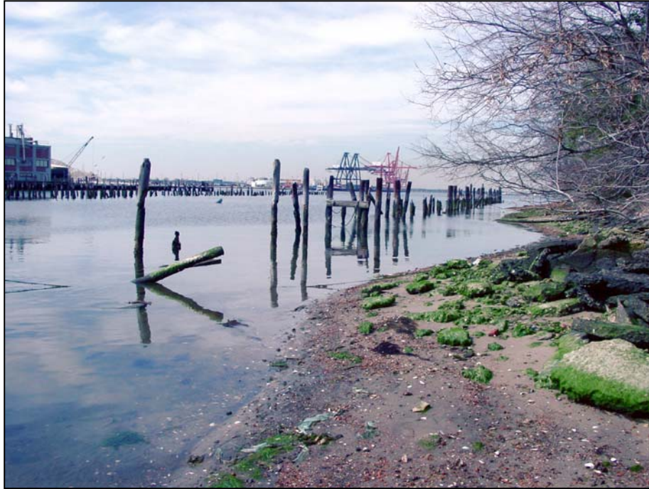
Timber Piles (Future River Clean-Up Area) South Side of Plum Point March 2002
